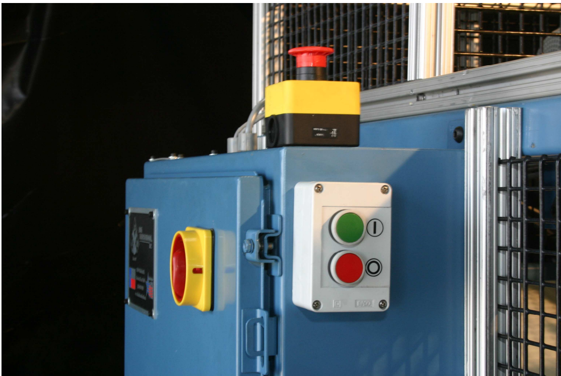
Figure 3.0 – Operator Start Station.
