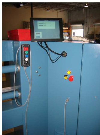
Fig. 2.2 Operator start stop station
